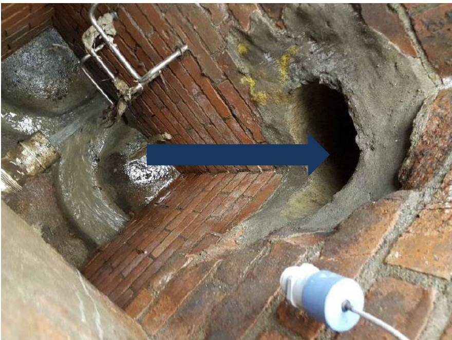
Figure 2-2 : COP showing high level overflow to stormwater (arrow), and water level monitor.
