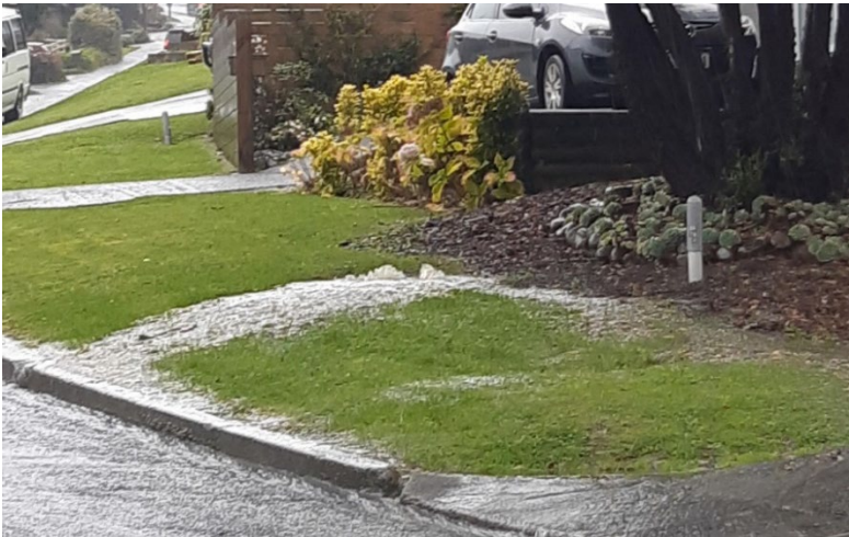
Figure 2-4: View of an uncontrolled overflow from a manhole into a nearby kerb and channel
