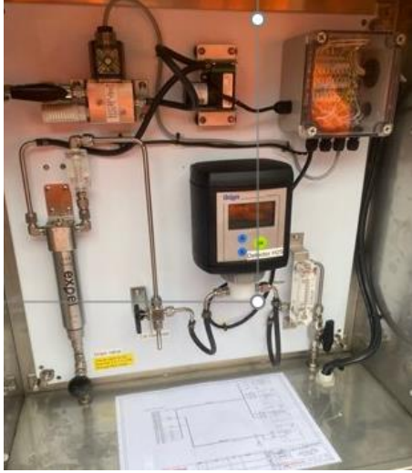
Installed H 2 S monitors in the inlet tunnel vent and milliscreen building air discharge stack
