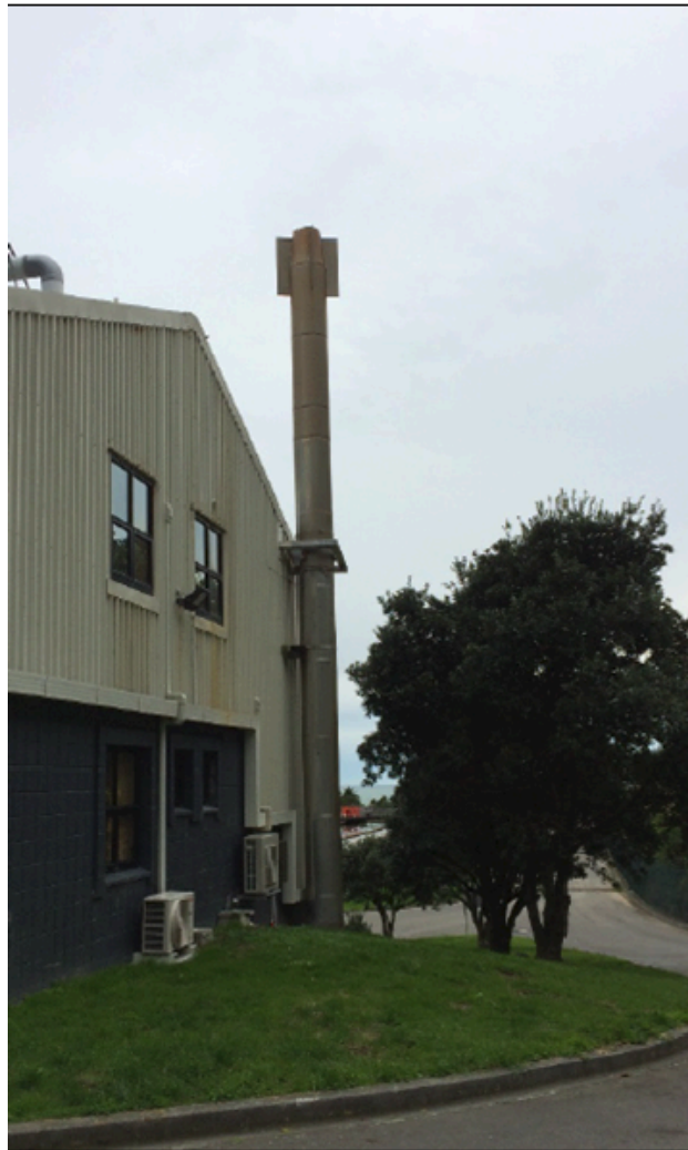
Figure 7. Milliscreen Building Discharge Stack
