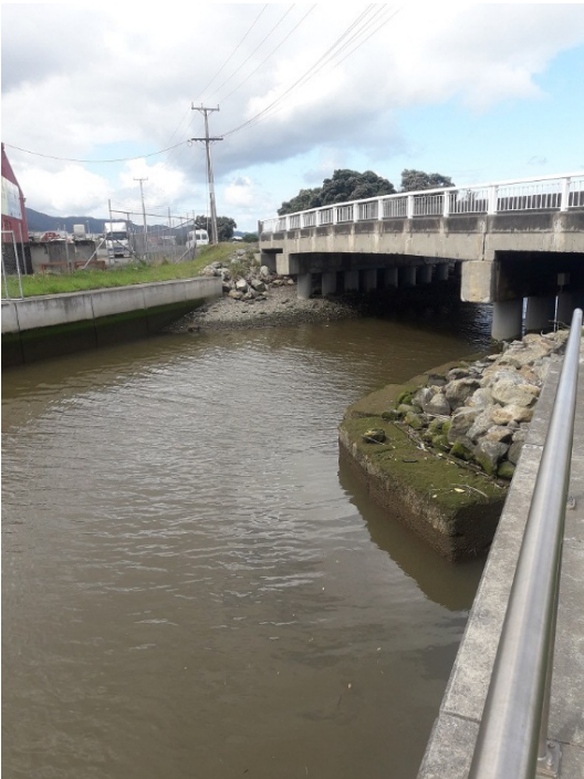
Figure E-28: Main plant overflow outlet on 12 November 2019
