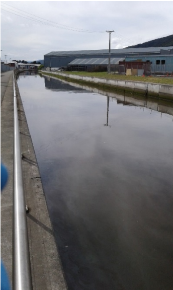
Figure E-51: Main plant overflow outlet on 30 March 2020
