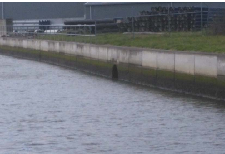
Figure E-63: Main plant outfall outlet on 06 June 2020
