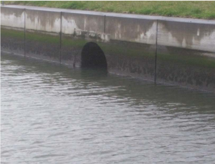
Figure E-77: Main plant outfall outlet on 21 June 2020
