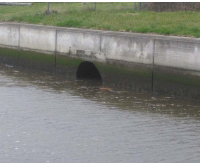
Figure E-73: Main plant outfall outlet on 20 June 2020
