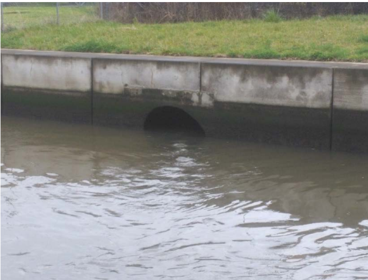
Figure E-69: Main plant outfall outlet on 19 June 2020
