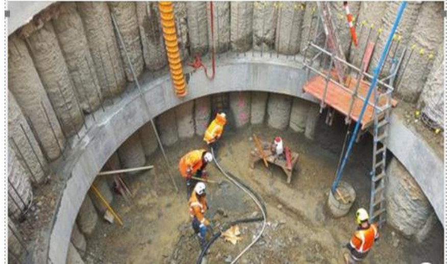
Work underway in the construction of the Taranaki Street Pumping Station. This project is part of the wider CBD wastewater network renewal programme in Wellington City, that will enable growth in the CBD as well as protect te Whanganui a Tara.
