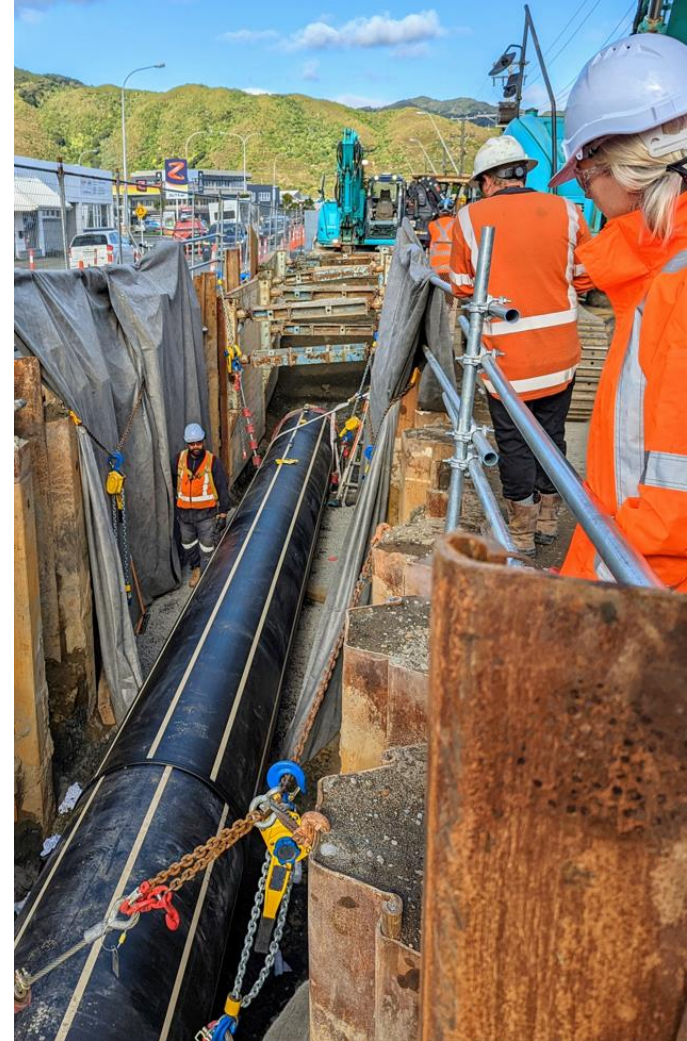
Working around underground services in complex locations has been a feature of the project to duplicate part of the wastewater main to Seaview Treatment Plant. GM of Network Strategy and Planning Julie Alexander (right) observes proceedings.
