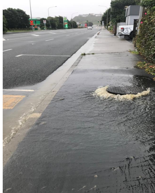
A wastewater manhole lid is pushed up from its base by an excess of water in the pipes. Rainwater enters wastewater pipes through faults and through connections to the stormwater network, built as a way to divert wastewater from houses in case of a blockage. These network discharges will be addressed over time, under new consents being drafted.
