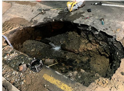
Pipe burst exposed
