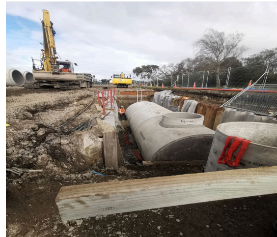
Donald St Pump Station in Featherston
