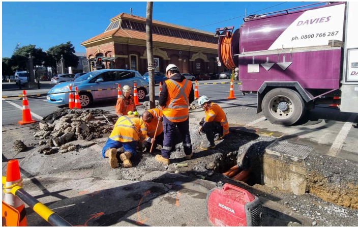
Crews busy repairing the burst water pipe on Customhouse Quay. Photo: RNZ/Krystal Gibbens
