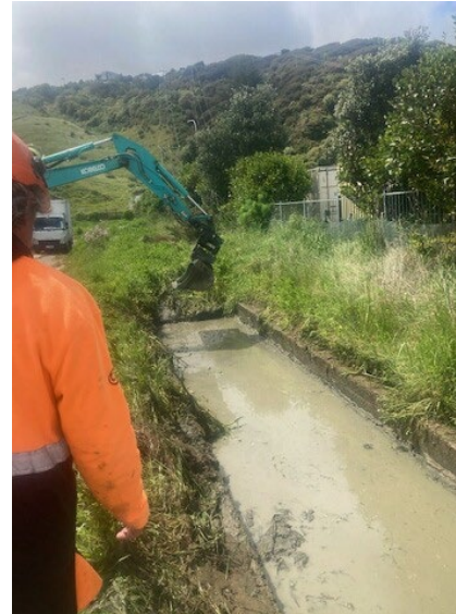
A Wellington Water crew clearing the stormwater culvert near James Street, Plimmerton
