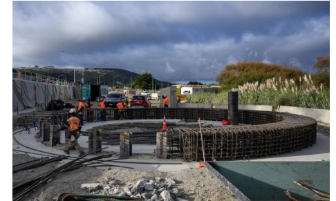
Sections of the new wastewater storage tank in Porirua being built. Once completed the tank will hold wastewater during times of heavy rain to reduce overflows into the environment.
