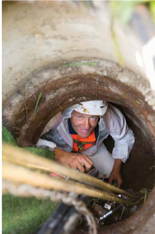
New lining being applied to a wastewater main in Titahi Bay, Porirua
