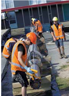
One of the Waterloo well-field pumps is readied to be put back in service after cleaning of the well
