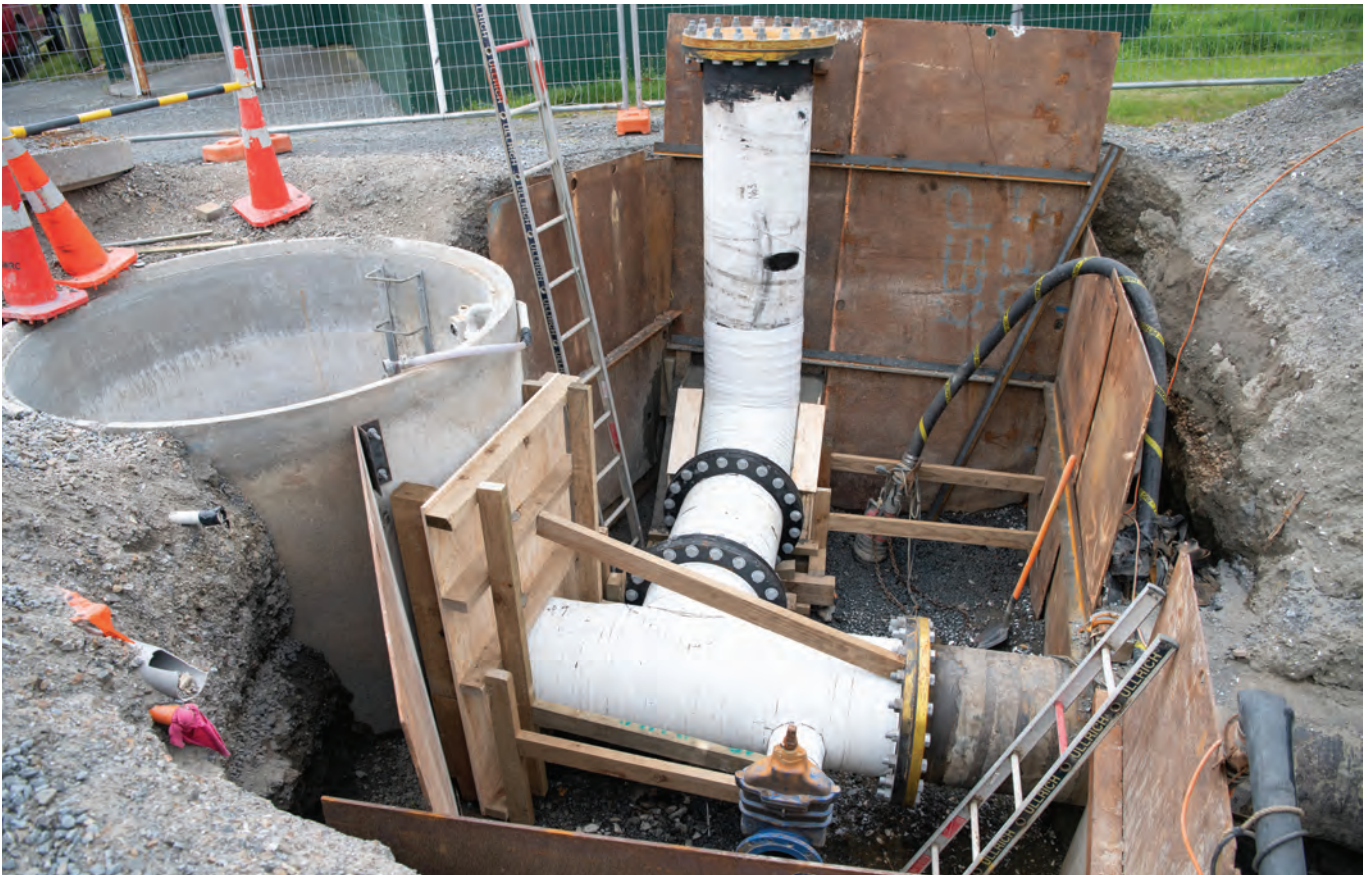
Installation of the UV treatment plant at Gear Island. Our water supply infrastructure is designed to operate regionally and doesn't supply each city on a stand-alone basis.
