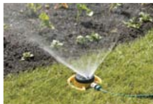
19. Sprinkler in garden
