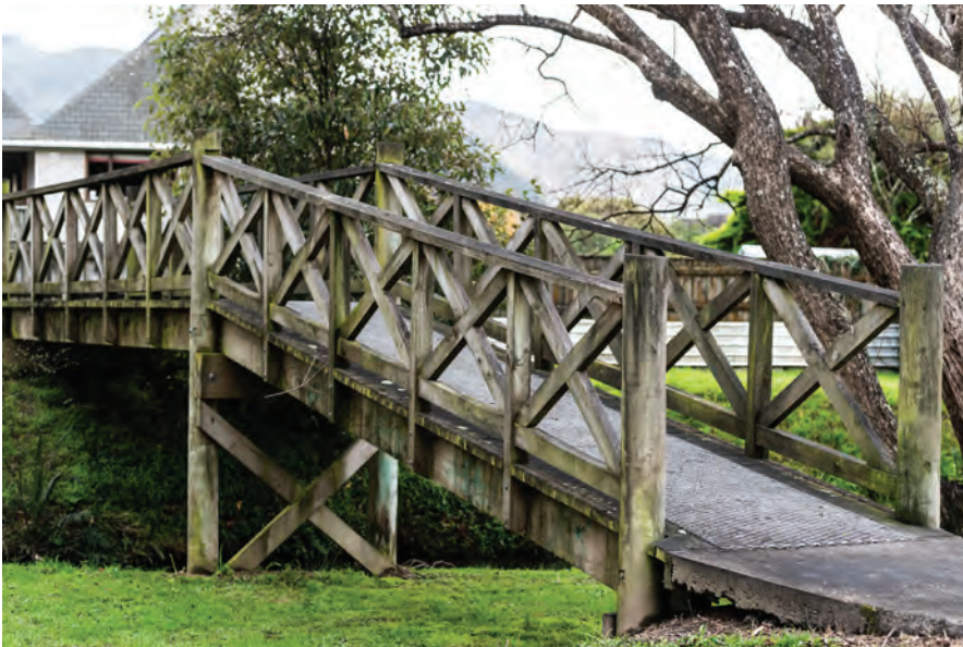
This older bridge at Willow Park will be replaced with a new bridge connecting with land purchased for the project at 4 Sunbrae Drive.
