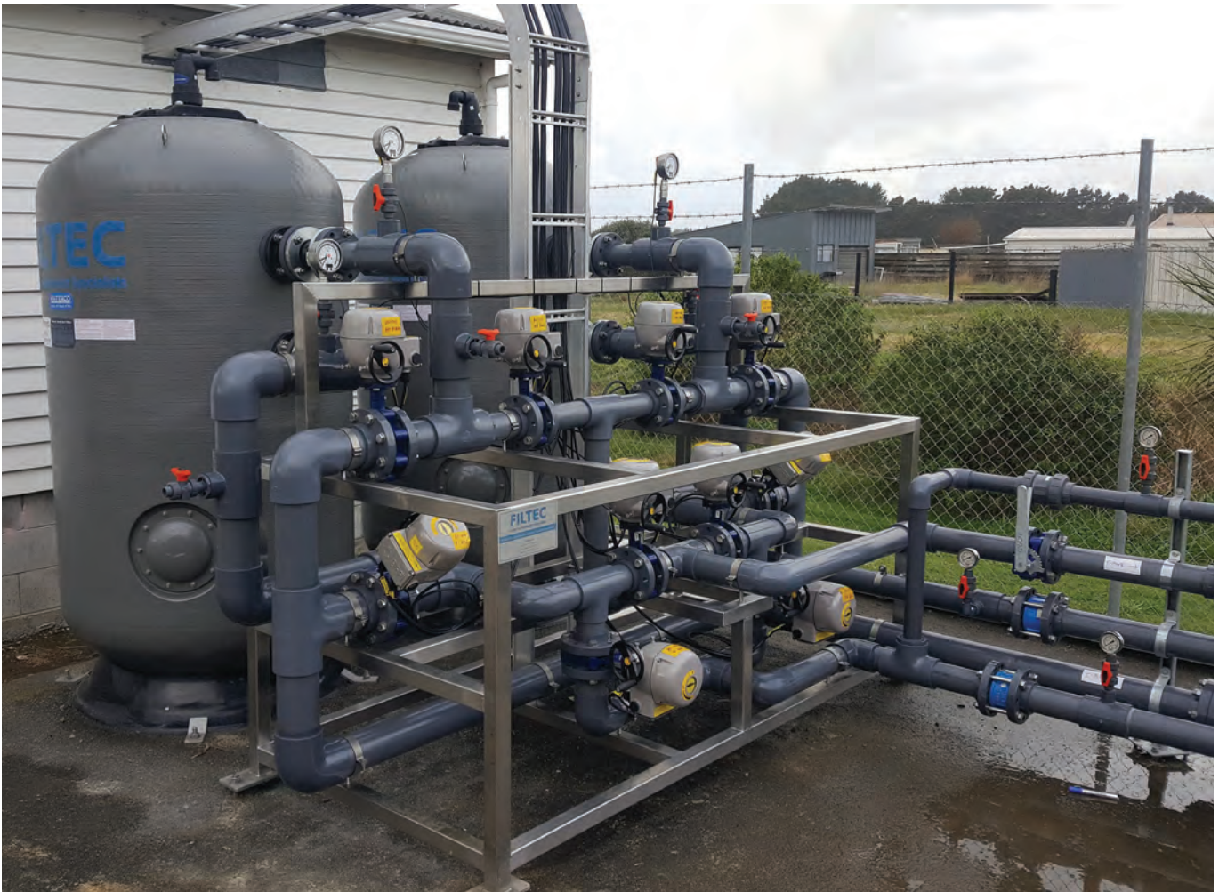
Filters similar to these will extract manganese from bore water supplying Martinborough, extending the ability to provide safe drinking water..
