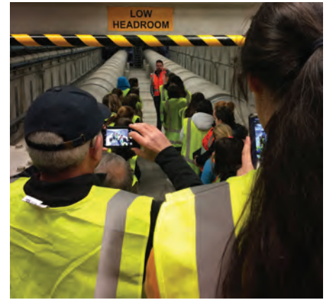
Massive pipes provide drinking water to the Wellington region.
