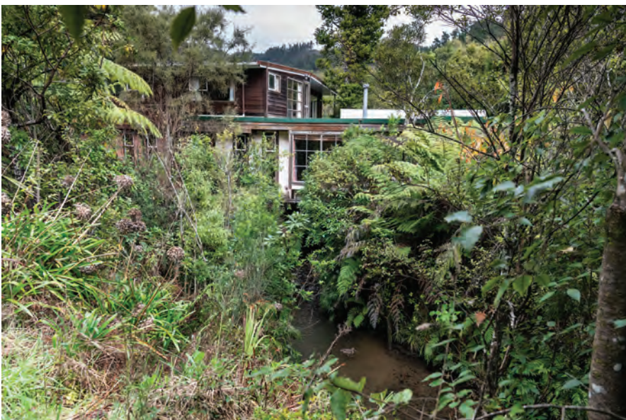
48 Blue Mountains Road – another project property. The house is built directly over the Pinehaven Stream.
