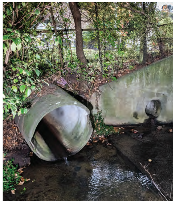
The culvert at the road crossing of Pinehaven Road and Blue Mountains Road will be upgraded too.
