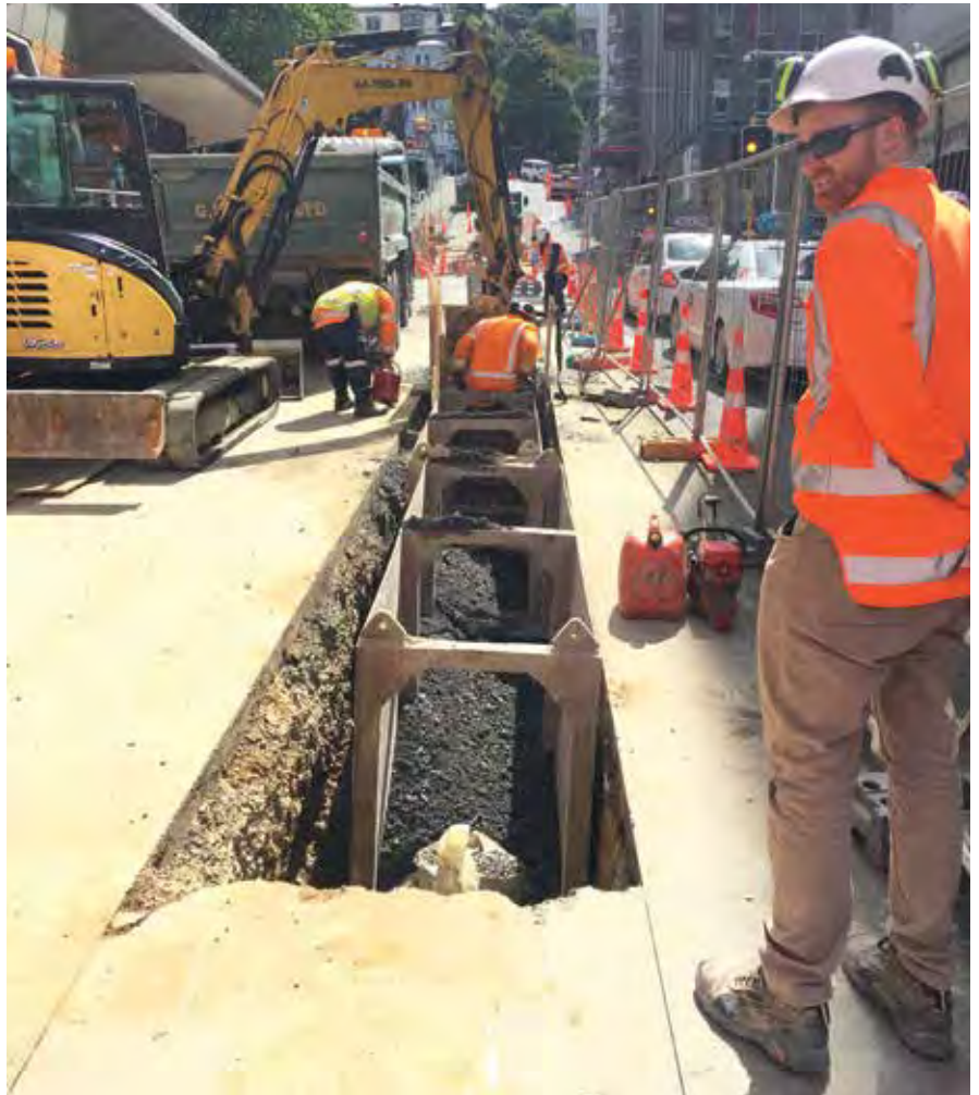
A worker on the Victoria and Dixon Street wastewater upgrade wearing full personal protective equipment (PPE) gear. Any person that enters a work site must be authorised and have full PPE.
