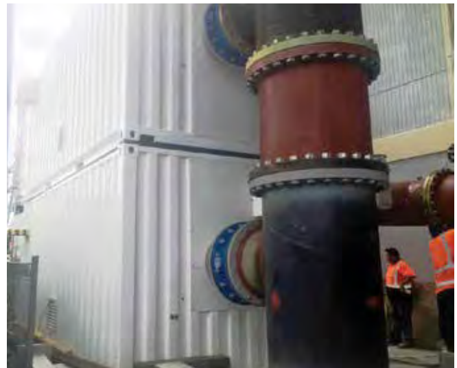
Ultra Violet (UV) kit installed at Waterloo Drinking Water Treatment Plant.
