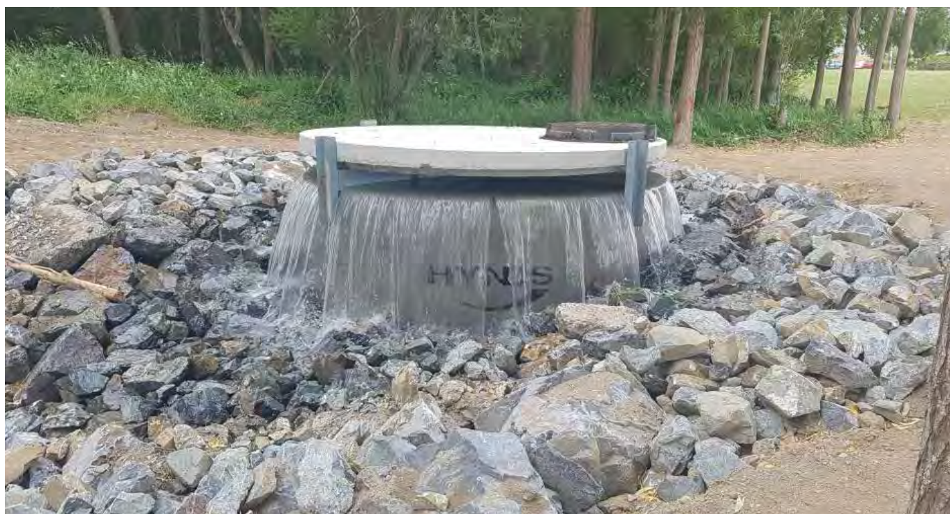
Water drawn from the Waiwhetu Aquifer flows into the Hutt River/Te Awa Kairangi from this pipe outfall. This water is unable to be treated by UV at the Waterloo Drinking Water Treatment Plant.
