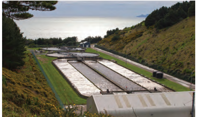
Porirua Wastewater Treatment Plant.
