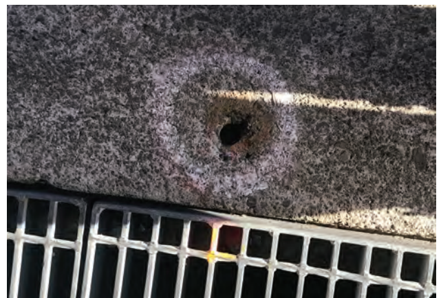
Point of injection in ground at Seaview Wastewater Treatment Plant.
