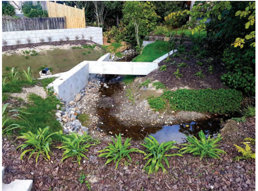
As part of the consent requirements, the Redwood Stream was reinstated to a 'natural state' as it provided a spawning habitat to some species including eels.
