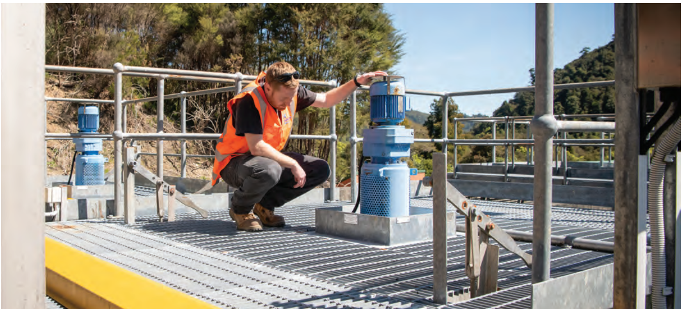
Steve checking over our equipment at Wainuiomata Water Treatment Plant.
