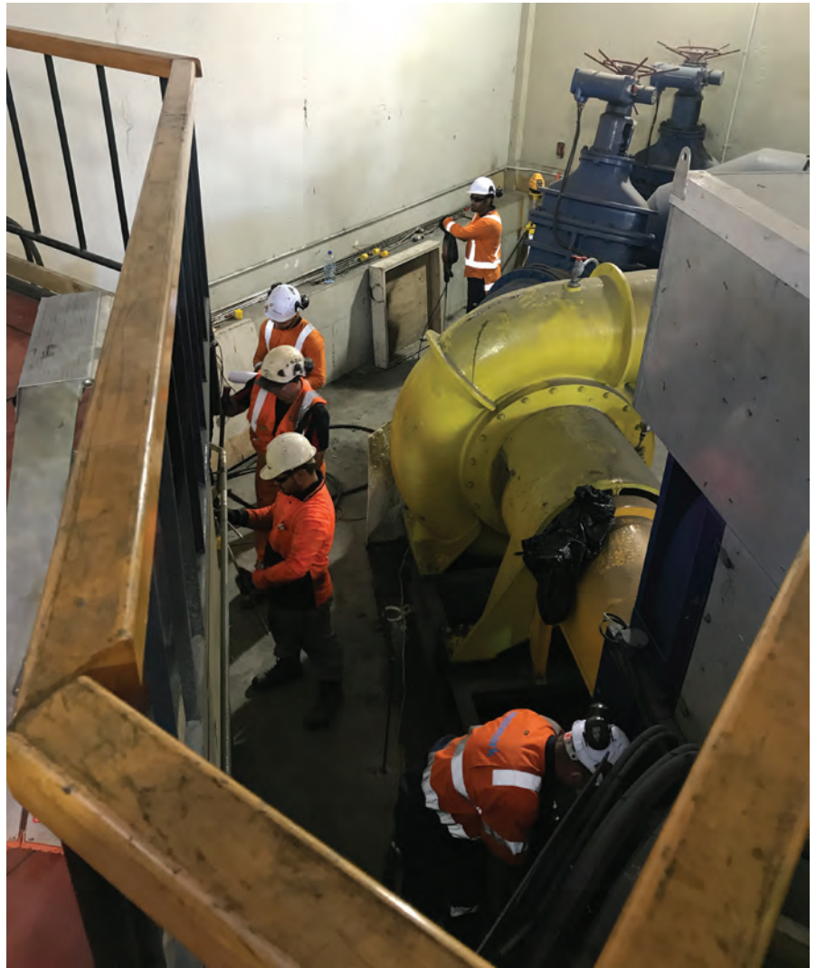
Mainmark team in the process of injecting resin through injection tubes 7m into the ground.
