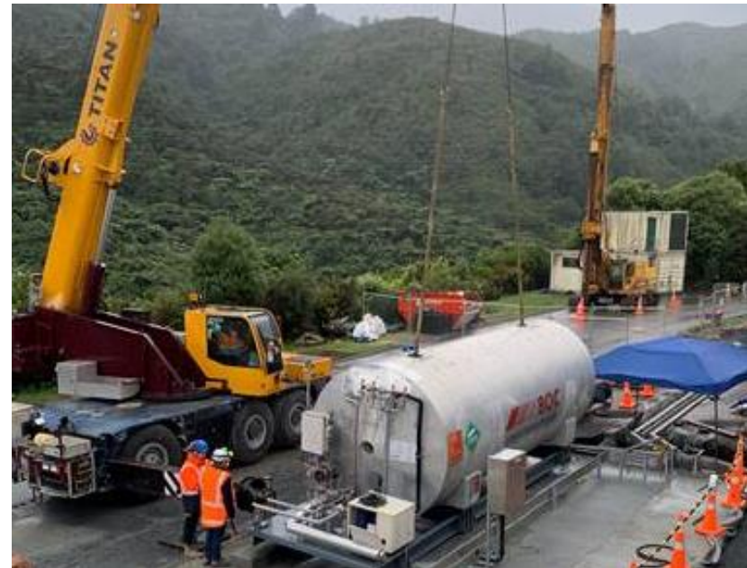
This new CO 2 tank at Te Marua Water Treatment Plant will allow us to start work on the dissolved air floatation (DAF) treatment system. DAF will help us to increase our treatment capacity by 60 million litres a day to a maximum of 140 MLD.
