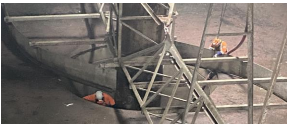
Workers clean out the bearing pit in a clarifier tanks at Moa Point Wastewater Treatment plant. The clarifier is now back online after failure of the bearing constrained the plant’s ability to treat water for several months. Above, the view from the tank floor.
