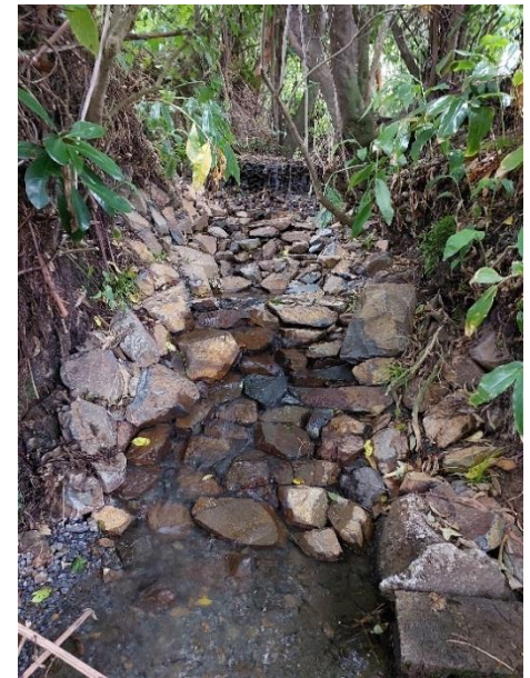
Before (above), the stream has eroded around poorly installed gabion baskets. Now (below), a rock cascade prevents further erosion of the stream bed and provides better fish passage
