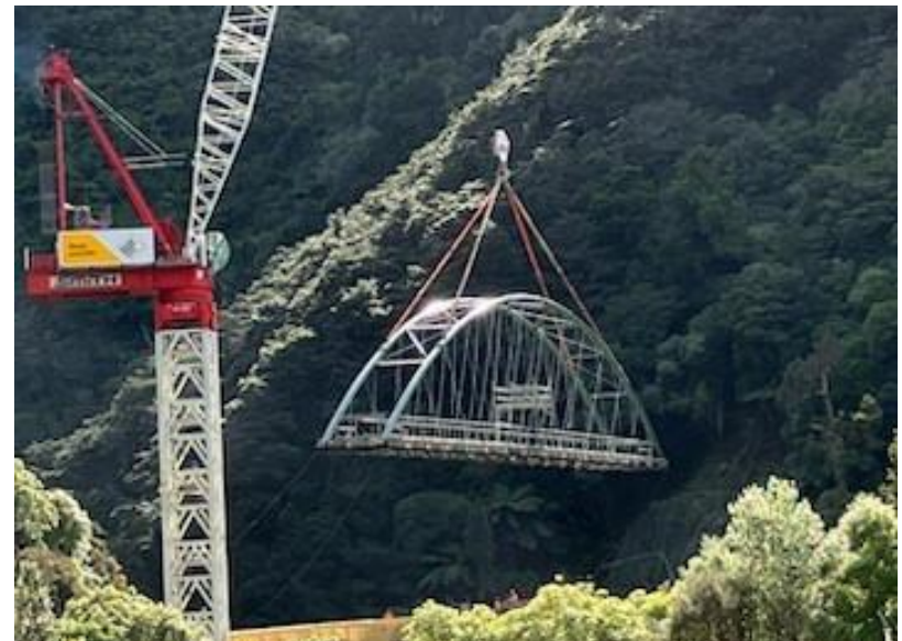
The Kaitoke Regional Park Arch bridge is lowered into place, to support a new pipe that will carry raw water towards Te Marua Treatment Plant. The new structure will improve water supply resilience in the event of a natural disaster.
