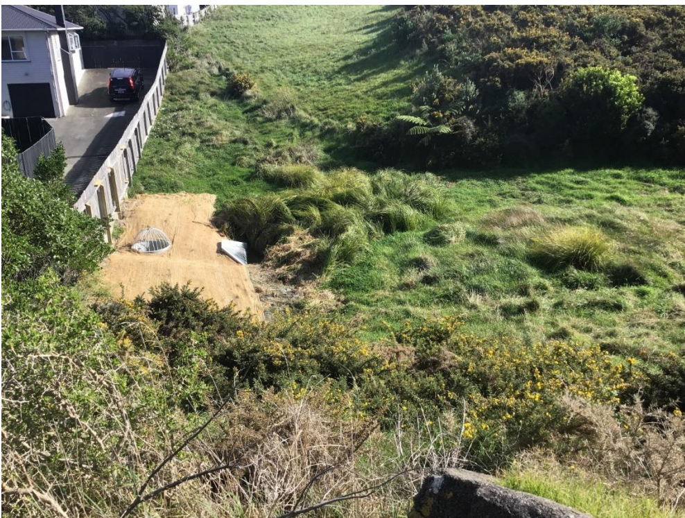
Image 5: The coconut matting covering the work space and the resulting repaired culvert
