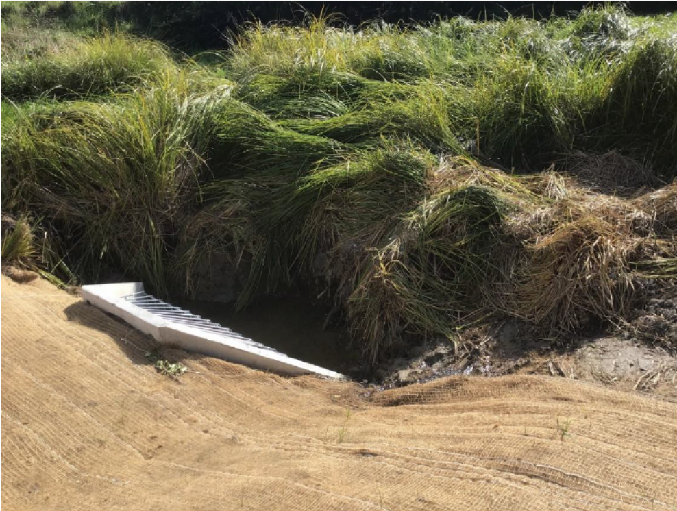
Image 6: The culvert inlet showing a pool (shaded) and carex overhanging the exposed dug out substrate
