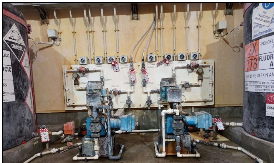
Figure 22 Gear Island WTP: Fluoride Dosing Pumps
