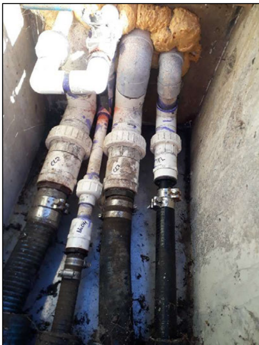
Figure 6 Te Marua WTP: Fluoride Dosing Point
