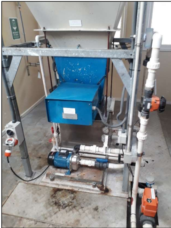
Figure 17 Wainuiomata WTP: Fluoride Feeder and Dosing Pump
