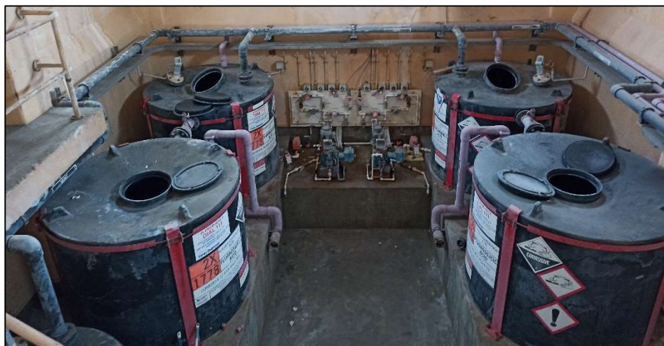
Figure 21 Gear Island WTP: HFA Storage Tanks
