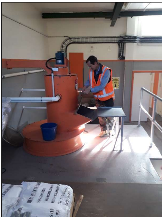
Figure 14 Wainuiomata WTP: SSF Powder Storage Hopper Loading Hatch
