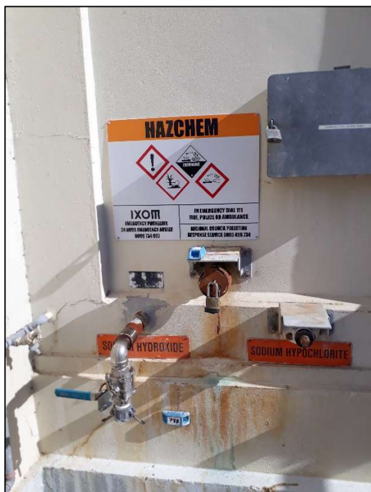
Figure 20 Gear Island WTP: HFA Tanker Delivery Connection Point (Centre)
