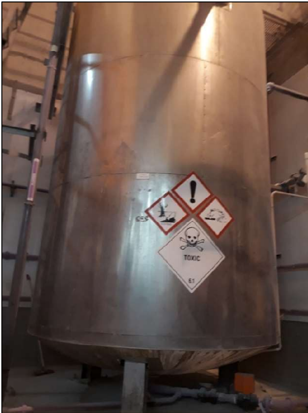
Figure 11 Waterloo WTP: SSF Day Tank
