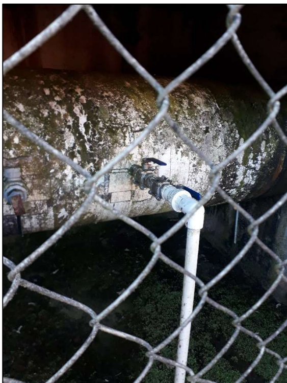
Figure 18 Wainuiomata WTP: Fluoride Dosing Point
