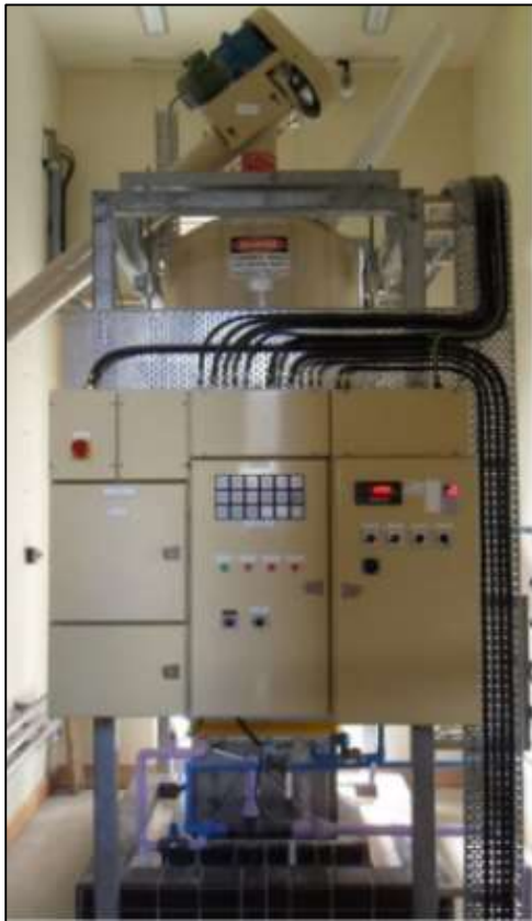
Figure 3 Te Marua WTP: SSF Day Hopper (Behind Panel)
