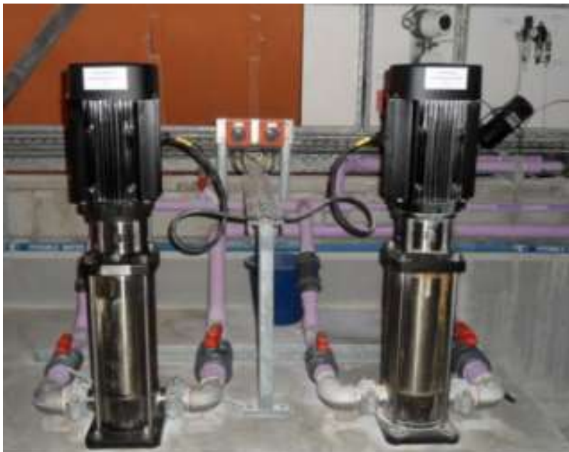
Figure 12 Waterloo WTP: Fluoride Dosing Pumps
