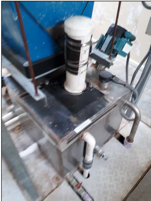
Figure 16 Wainuiomata WTP: SSF Mixing Tank
