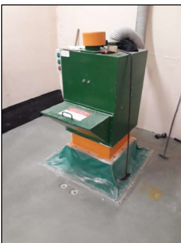
Figure 8 Waterloo WTP: SSF Powder Feed Hatch (Storage Hopper below Floor)
