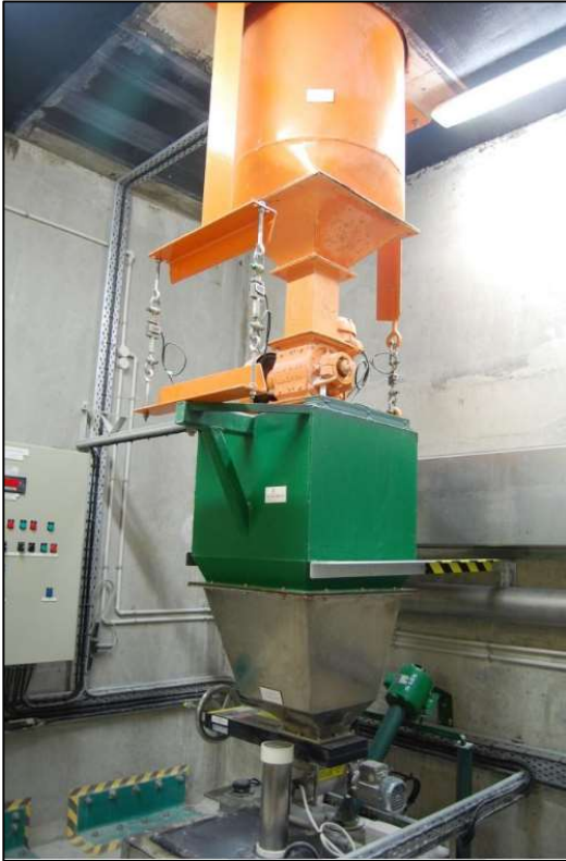
Figure 9 Waterloo WTP: SSF Powder Storage Hopper (upper) and Day Hopper (lower)
