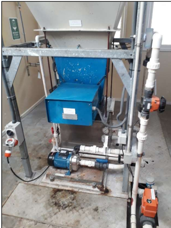
Figure 17 Wainuiomata WTP: Fluoride Feeder and Dosing Pump
