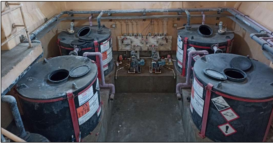
Figure 21 Gear Island WTP: HFA Storage Tanks
