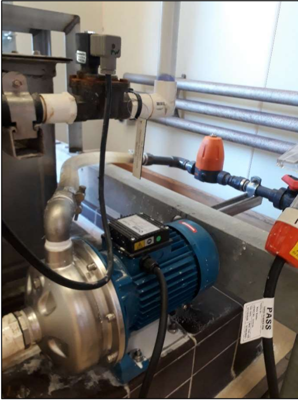
Figure 5 Te Marua WTP: Fluoride Dosing Pump
