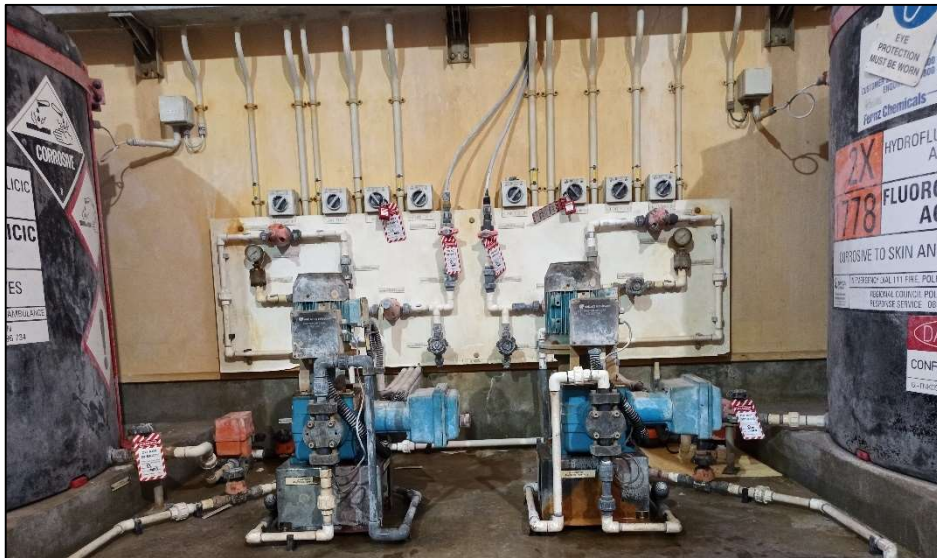
Figure 22 Gear Island WTP: Fluoride Dosing Pumps
