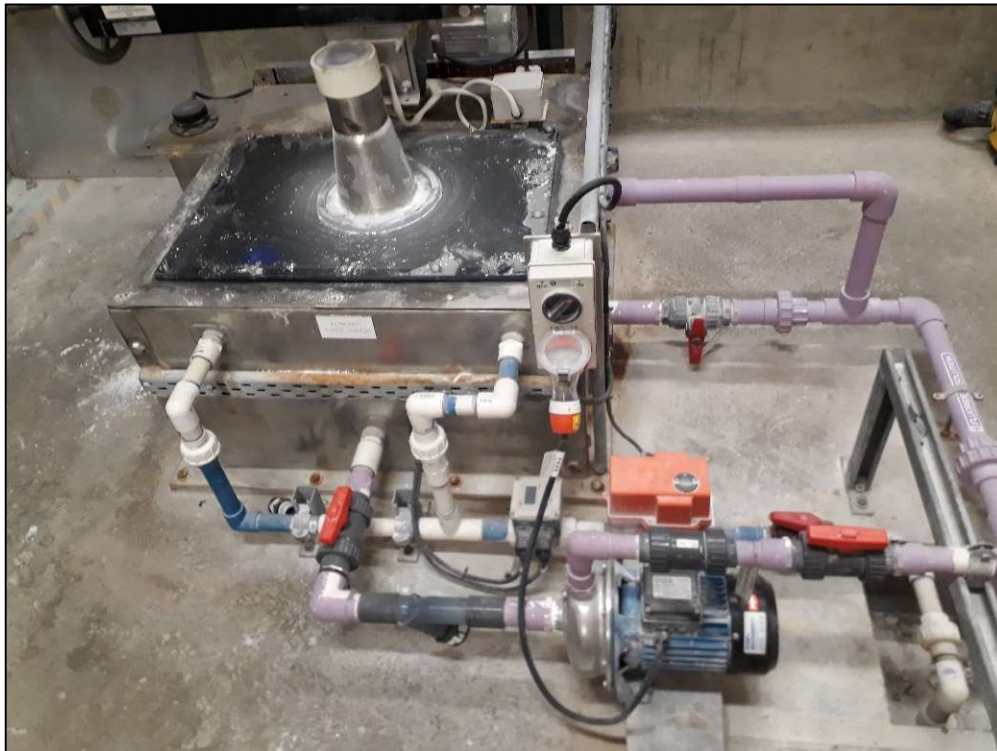
Figure 10 Waterloo WTP: SSF Mixing Tank and Transfer Pump
