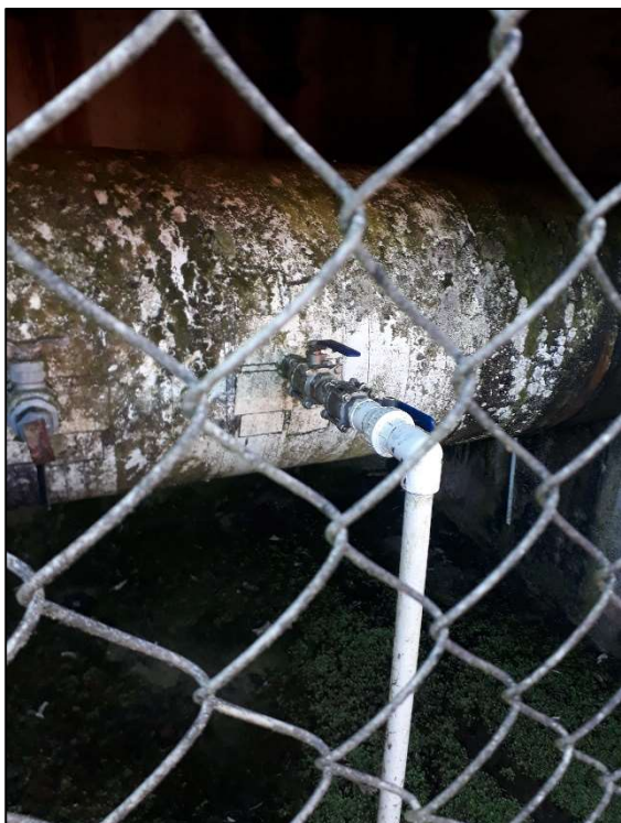
Figure 18 Wainuiomata WTP: Fluoride Dosing Point
