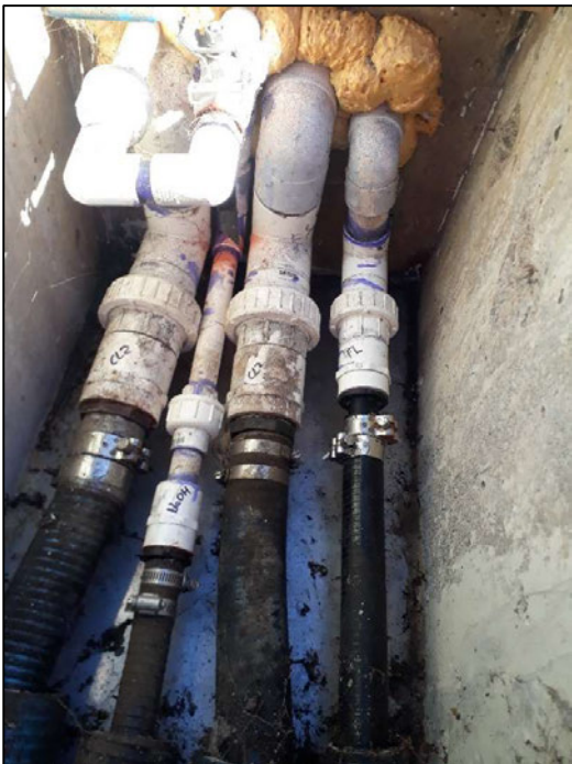
Figure 6 Te Marua WTP: Fluoride Dosing Point
