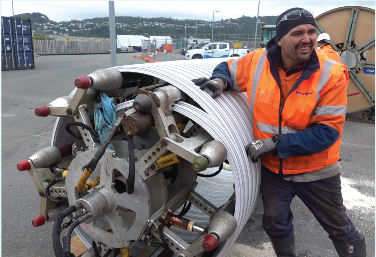
An above-ground demonstration of the pipe-lining machine showed how the plastic compound spirals forward and is glued into place as it advances through the host pipe.
