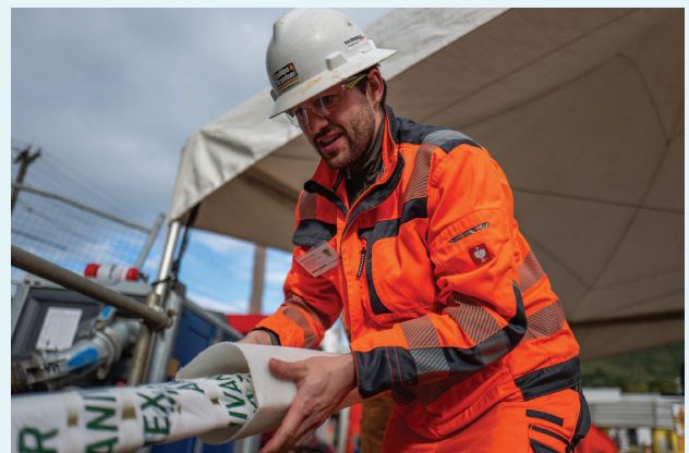
The pandemic delayed the manufacture and installation of the liners made in Germany to repair the Mt Albert tunnel sludge pipes.
