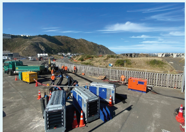
Pumps and temporary piping were used to bypass the corroded section of pipe while it was lined.
