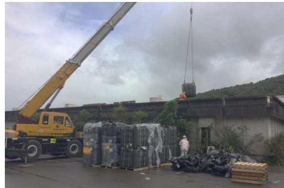
Carbon granules are dropped into filtration tanks at Te Marua, Upper Hutt.
