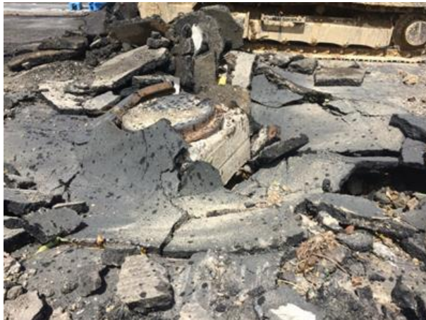
A pressurised stormwater main blew out in Lower Hutt
