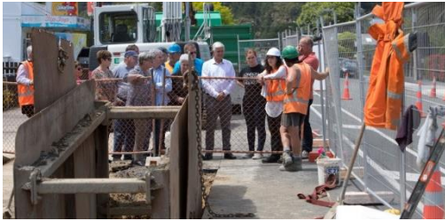
Following local body elections in October, we organised a visit for new councillors (and old ones) to water treatment plants and a pipe renewal project. More pics page 12.
