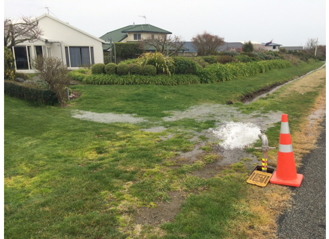
The water supply network was flushed clean by opening 14 hydrants at locations set by our modelling team
