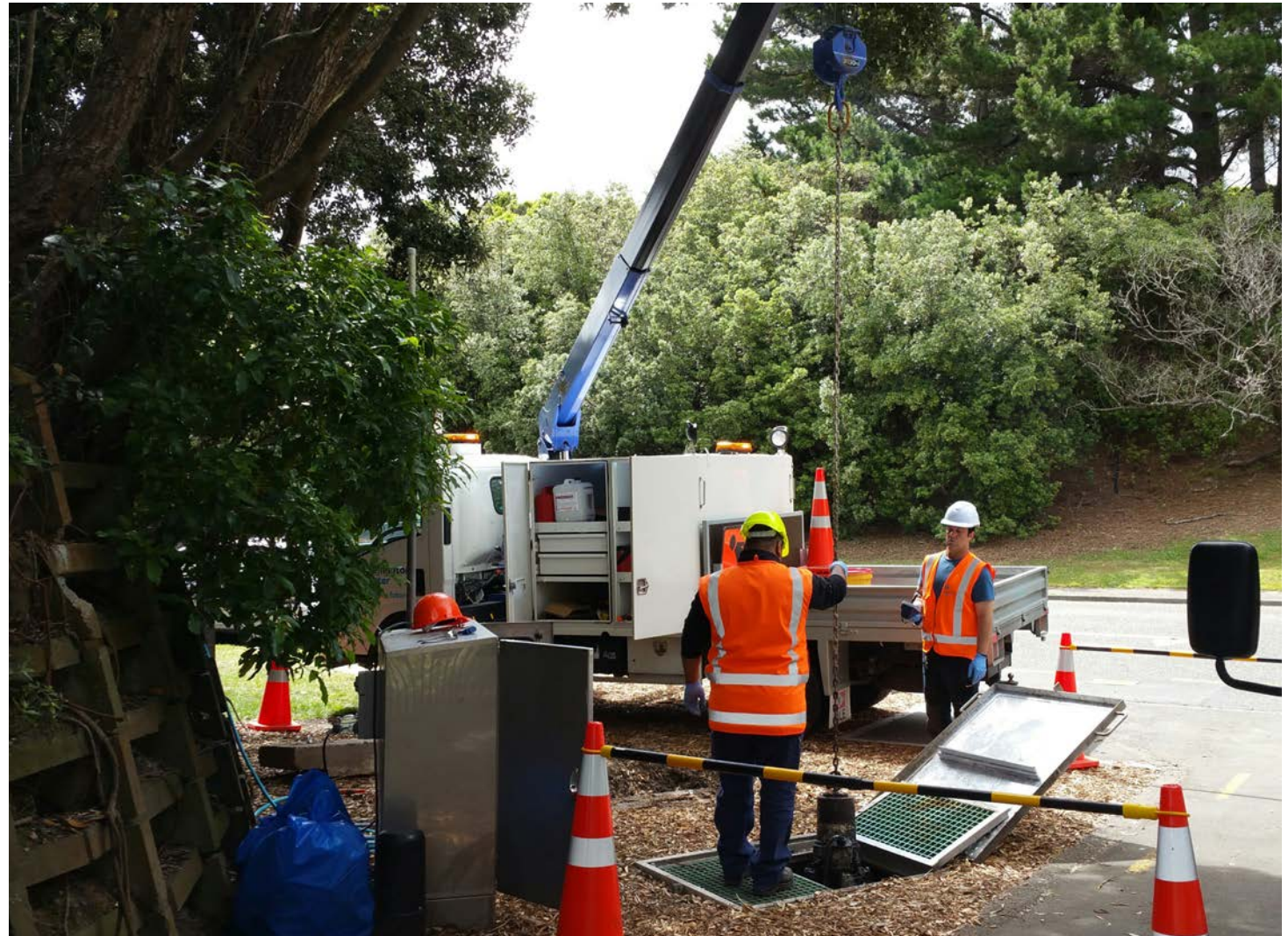
Wellington Water staff pull a pump out of wastewater pumping station for inspection
