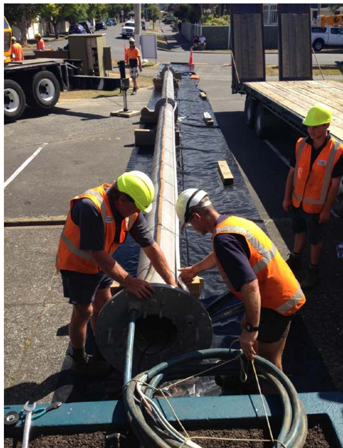
After the Waterloo well affected by iron bacteria was cleaned, the bore's pump is attached to a 16m positioning pipe in order to be lowered back into the aquifer.
