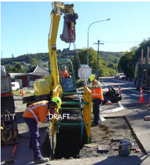
Workers lower shoring components into a trench for a project in Upper Hutt. The trench heights at which shoring must be in place have been reviewed by Wellington Water recently, to ensure workers performing tasks below ground level are safe.
