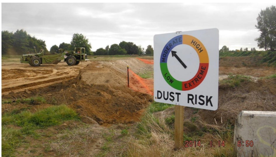
Photo 9 Dust risk signs will assist with communicating the risk to construction staff
