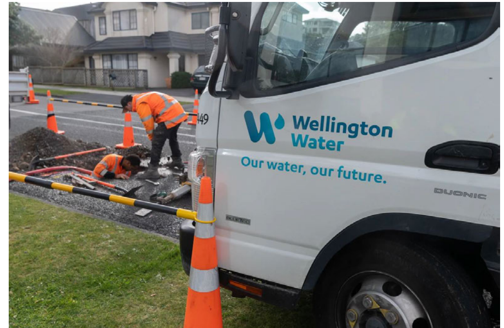
Ageing networks break down more often, requiring more reactive repairs
