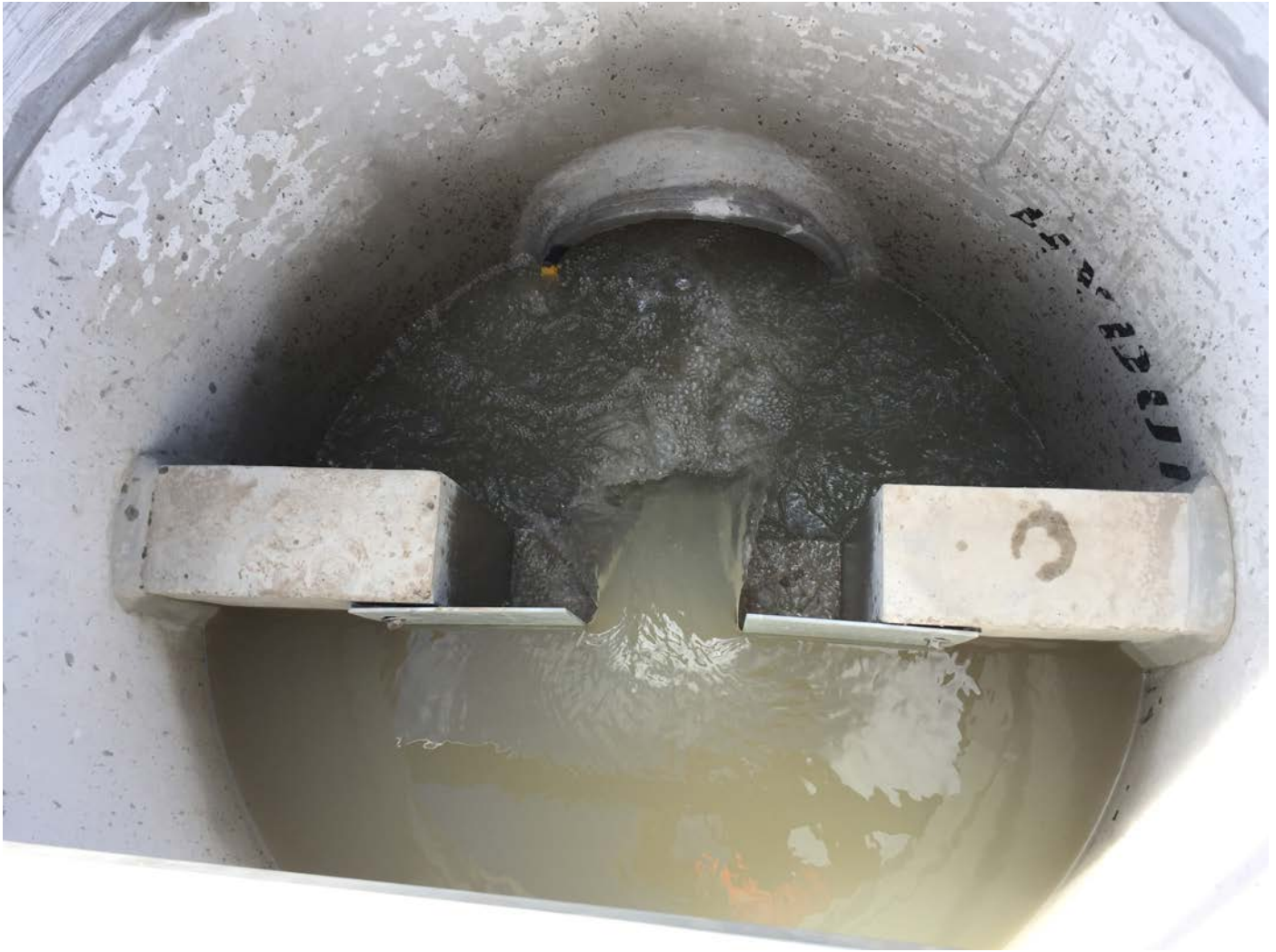
Figure 18: Outlet from wetland with weir plate controlling drawdown flowrate and operating water level.
