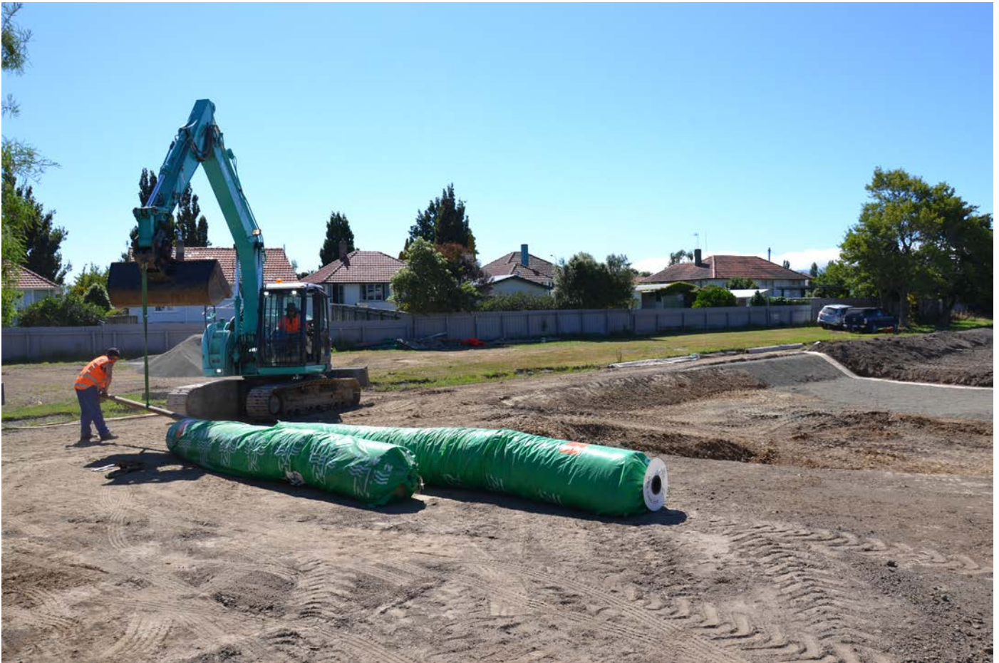
Figure 19: Installation of Geosynthetic Clay liner with bedding sand beneath and topsoil over.
