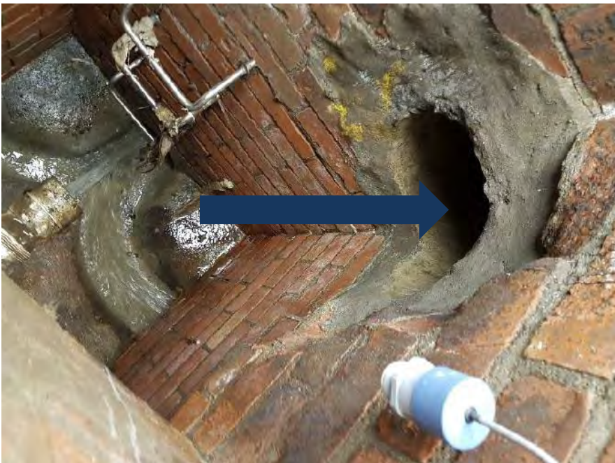
Figure 2-3 : COP showing high level overflow to stormwater (arrow), and water level monitor.
