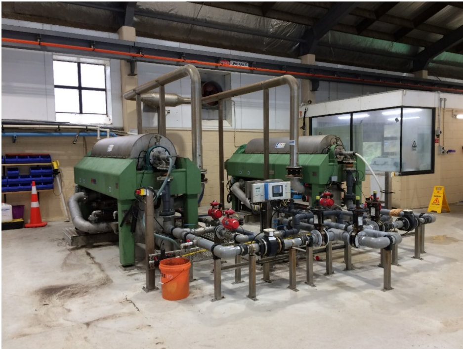
Figure 9: Sludge dewatering centrifuges
