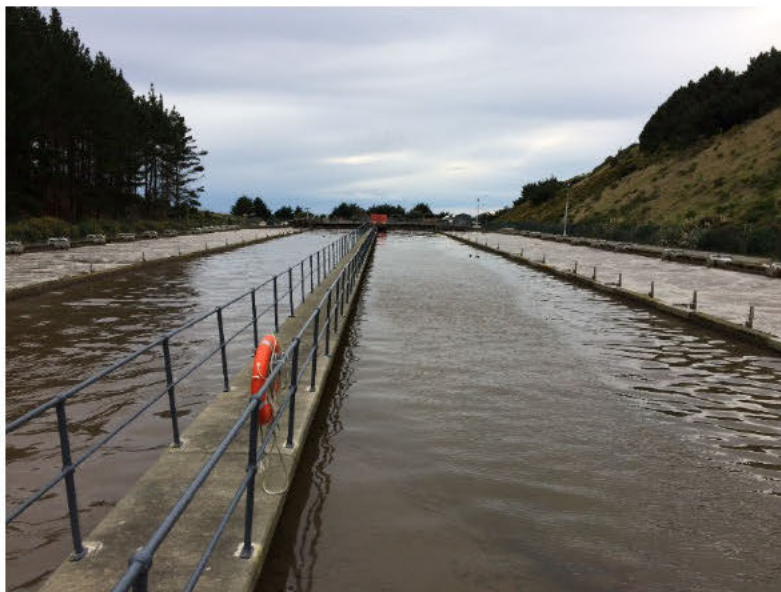
Figure 11: Aeration basin, with turbulence from active aeration being apparent in the side channels
