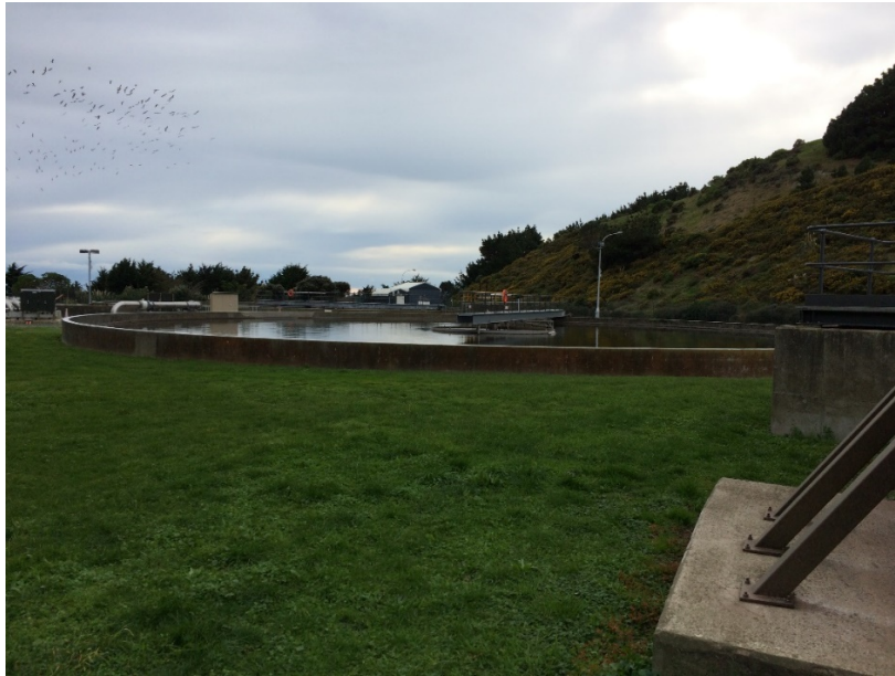
Figure 12: One of the three clarifiers used to settle remaining solids from the wastewater effluent prior to UV treatment and subsequent discharge via the ocean outfall
