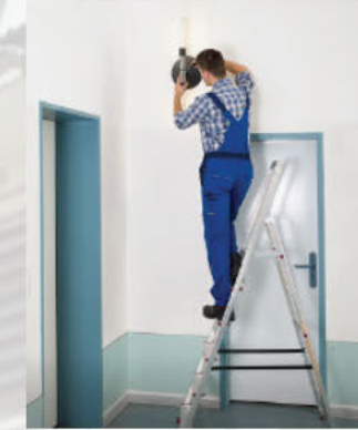
Incorrect Steps are side-on to the work activity
