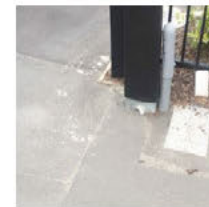
Water meter cover
